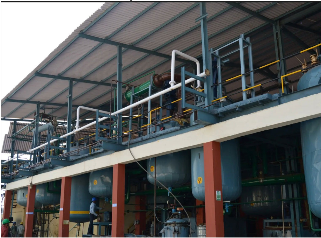
Reactors in Plant 3
