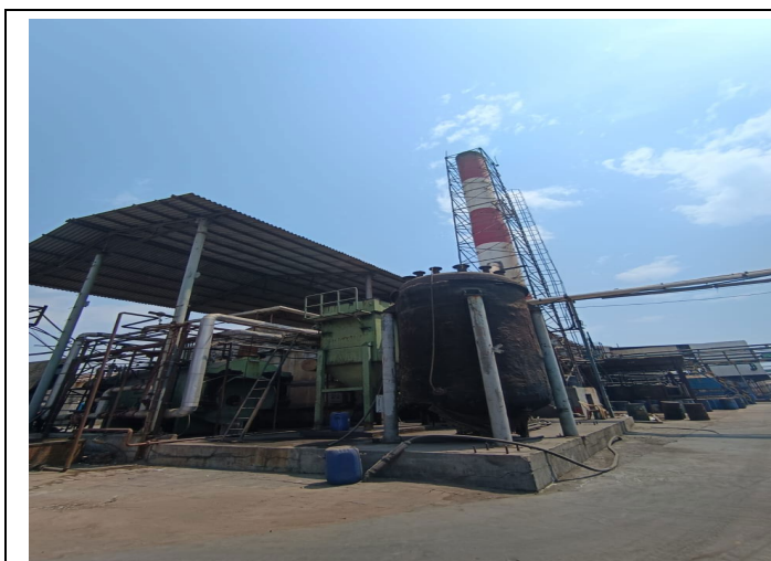
Boiler house consisting of Boiler and Thermic fluid heating system
