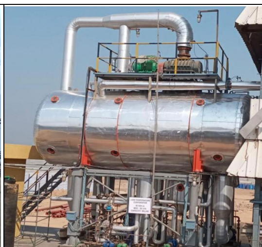
MVR_ waste water treatment facility
